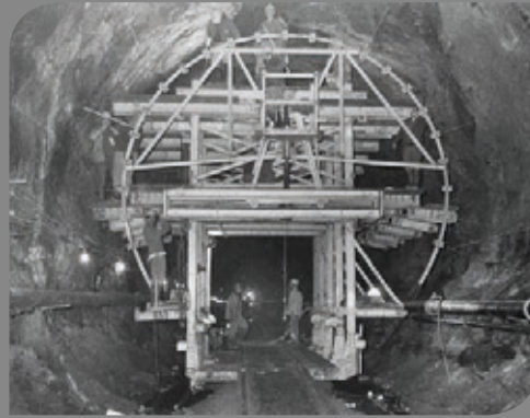
1 The world's longest tunnel carries water 170km to New York City from the Delaware River in the United States.
